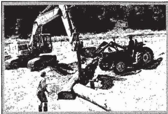
Photograph 3. NAMBUCCA RIVER, NSW. The construction of a log sill to recreate the pool/riffle sequence in a highly degraded sandbed river. NAMBUCCA River Stabilisation Task Force.
