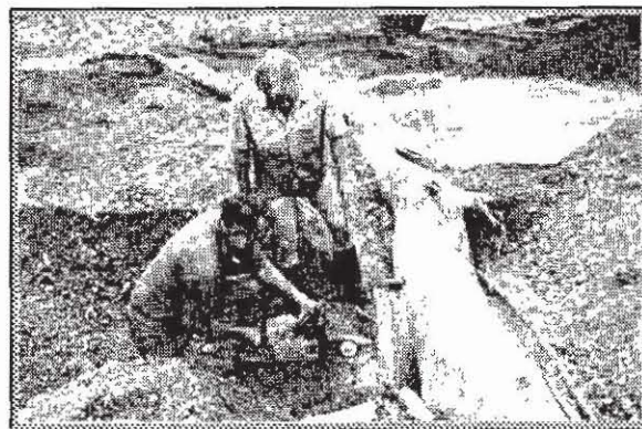
Photograph 5. Securing log sill timbers to vertical piles with friction pins. Banks of the stream are subsequently planted out with trees.
