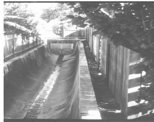
Figure 2 : A dry Powells Ck. urban stormwater channel at Strathfield
