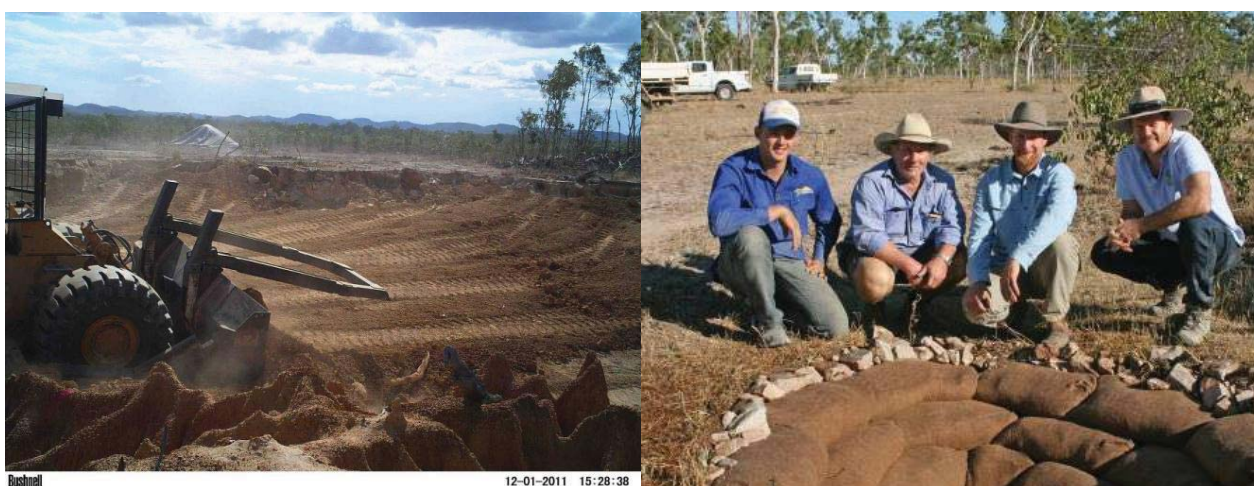
Figure 2 Left – An example of intensive gully regrading in the Normanby catchment (Jeff Shellberg) and (right) small scale gully control works in the Burdekin catchment (courtesy Nth Qld Dry Tropics)..
