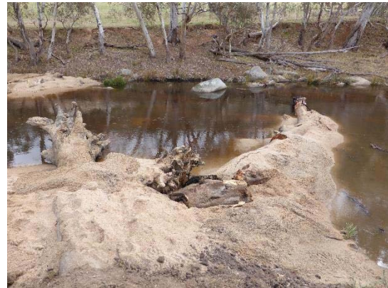
Figure 8. Upstream angled groyne on left and raised downstream angled groyne on right
