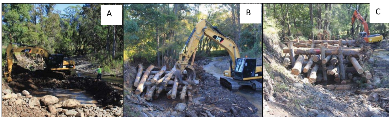
Figure 5 - Construction of ELJ, (A) the pit dug into the creek, (B) placement of logs, (C) completed ELJ
