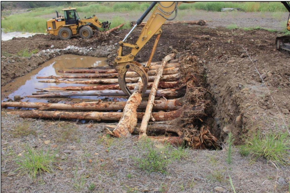
Figure 3 - Precise placement of logs to create the log jams in the Warrill Creek
